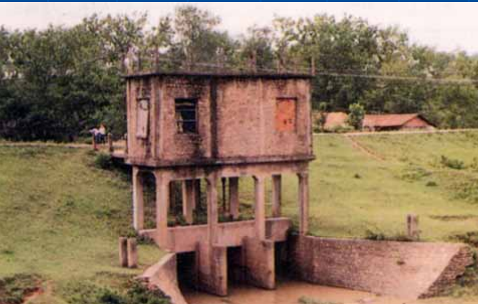
Floodgate of three hole
